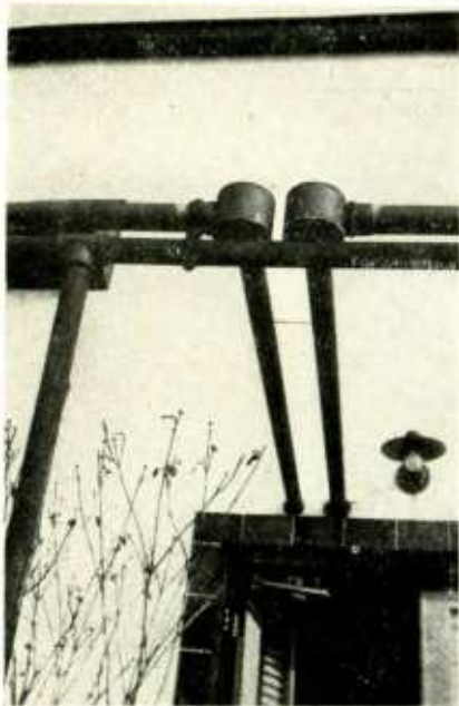
Fig. 3. Showing method of handling elbows in concentric lines to allow for contraction and expansion
